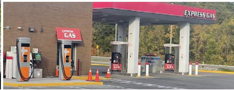
Level 3 EV Chargers installed at Express Gas in Akwesasne funded by the ICE's Charger Up program.
